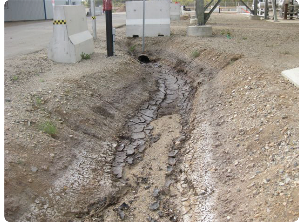
Sediment and soil erosion were perpetual problems at this industrial location.
