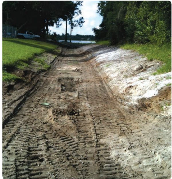
This residential stormwater channel would flood during heavy rainfall events.
