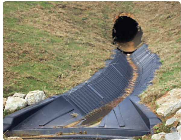
SmartDitch will self-cleanse itself of minor sediment build-up during a typical rain event.
