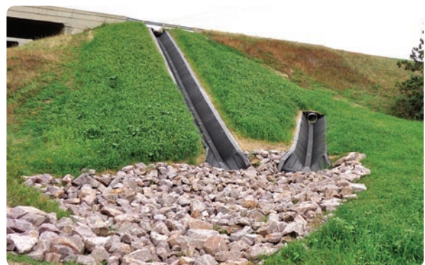
Portage, WI After: SmartDitch replaced the old Riprap, improved drainage, and eliminated erosion.
