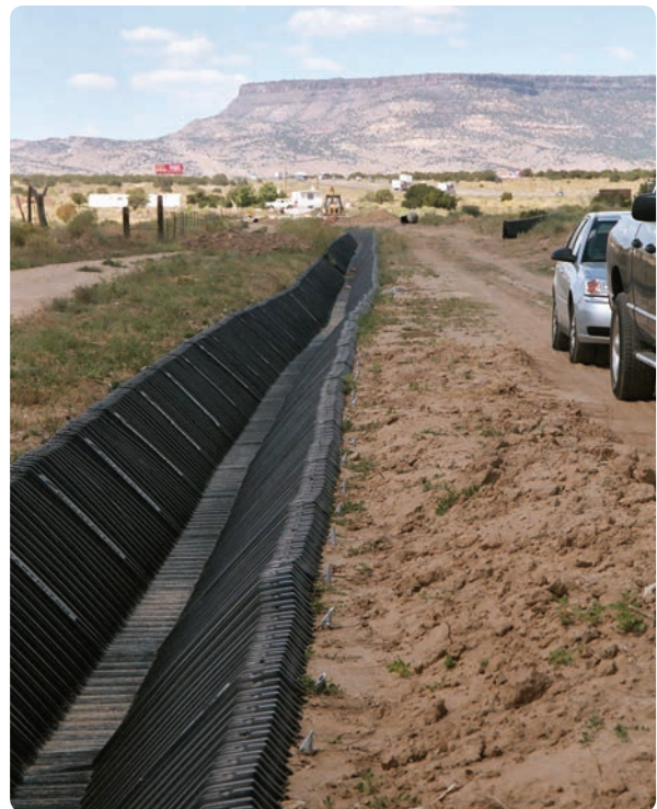
SmartDitch delivers more than 90% of all water from the original source.
