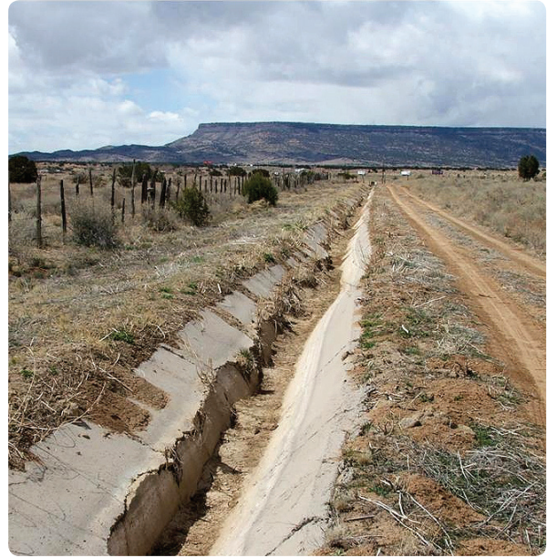
Cracked concrete irrigation ditches present major problems in rural farming communities.
