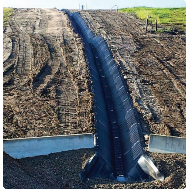
SmartDitch controls stormwater overflow coming from landfill caps.
