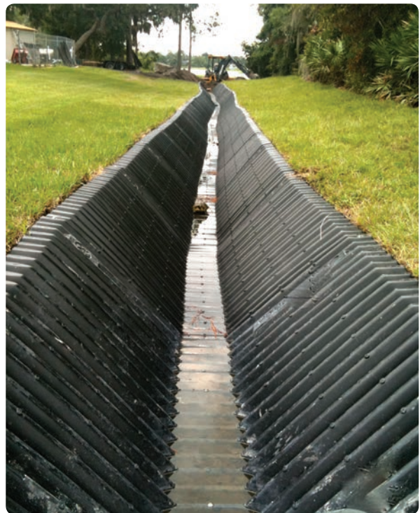
SmartDitch replaced the poor performing channel, improved flow, and required less space.
