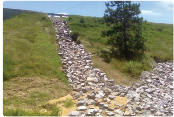
Portage, WI Before: Riprap continued to fail at this DOT drainage outfall.
